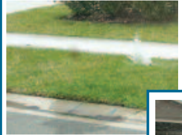
Small geyser caused by a broken sprinkler head
